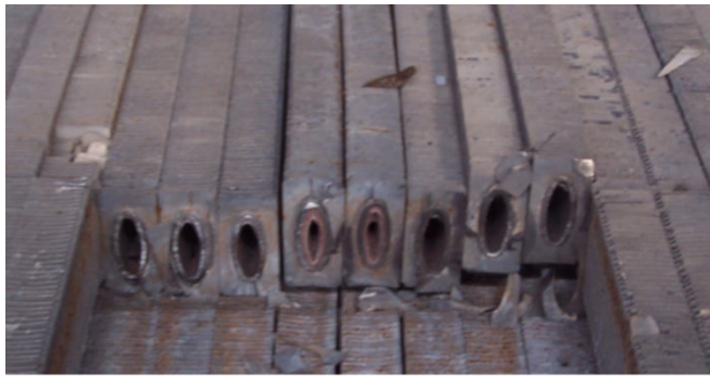
Fig. 26. Boiler scale observed in tubes of heat exchanger
