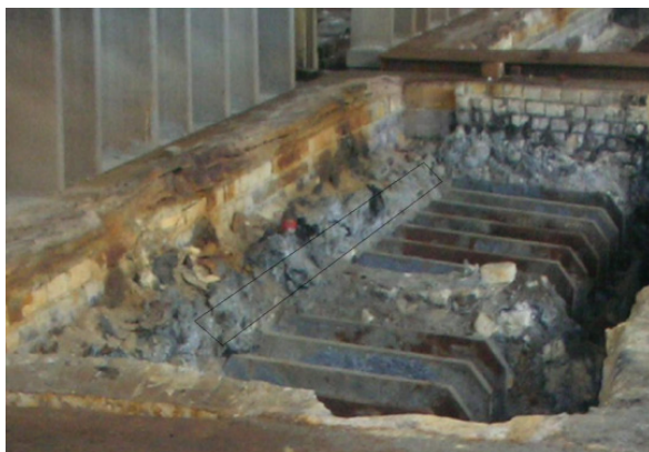
Fig. 19. Damaged back wall of an industrial magnesium electrolyzer due to the frequently washing of the small electrolyte circulation
